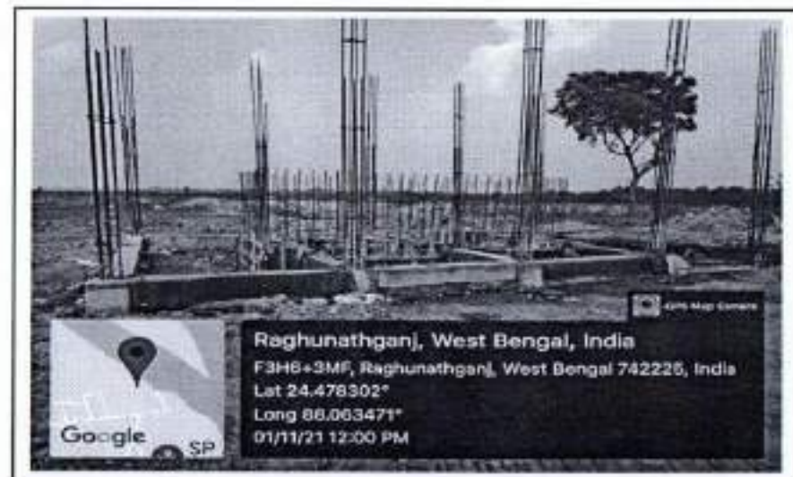
CHLORINATION -RAGHUNATHGANJ STP
